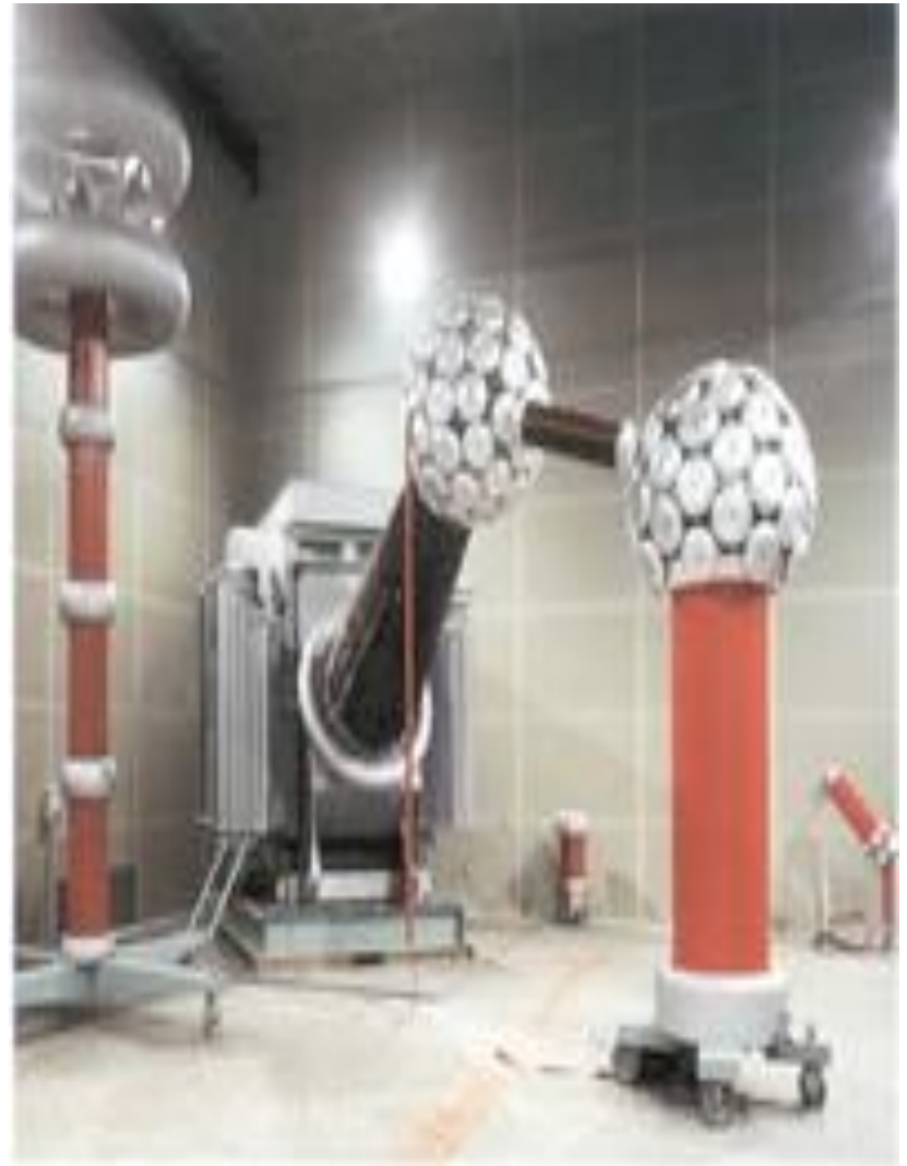
Single metallic body (DC Generator 900 kV)
