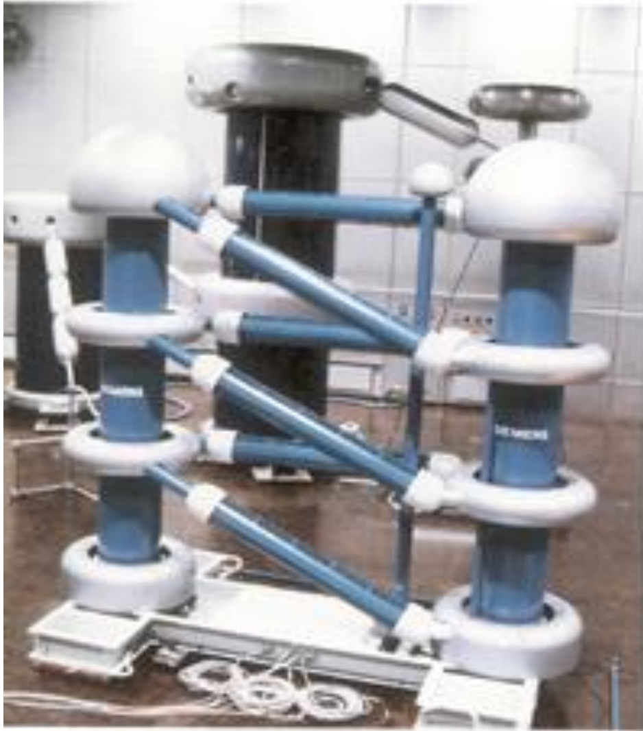
Segmented electrodes(Complete HV lab (600 kV AC))
